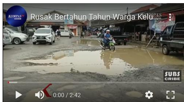
Figure 1.2 Damaged Road Condition (Source: Kompas.com, 2021)
