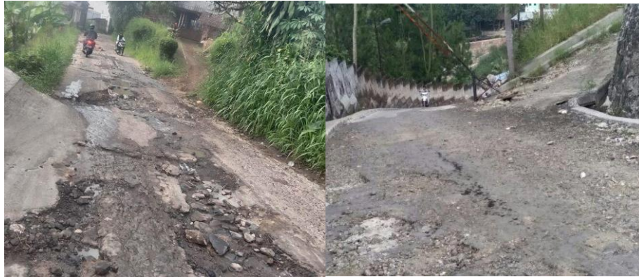
Picture: Road Conditions that are Still Damaged on Jalan Lewi Nanggung, Cicurug District, Sukabumi Regency
